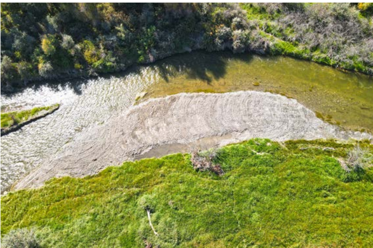
Photo 3. Deep pool feature with adjacent gravel bar constructed on African Queen channel (post-construction, 3006 cfs)
