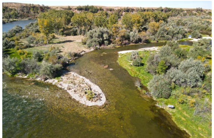
Photo 8. Narrowed entrance at African Queen channel w/apex debris jam installed to induce flow split (post-construction, 2866 cfs).
